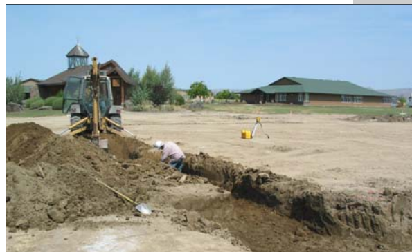
A view from the soccer field of the foundation prep for the new Science Center (southwest corner).
